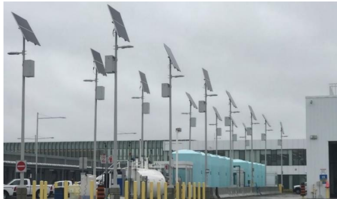
Figure 11 Solar-Powered Lighting System installed at Williams Parkway Operations Centre
