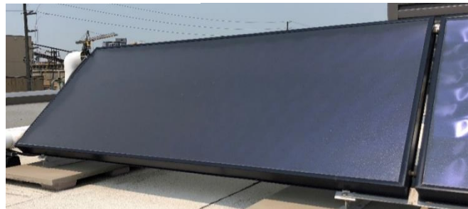
Figure 10 One of four solar collectors that are a part of the solar thermal system installed at Brampton Apparatus and Maintenance Facility
