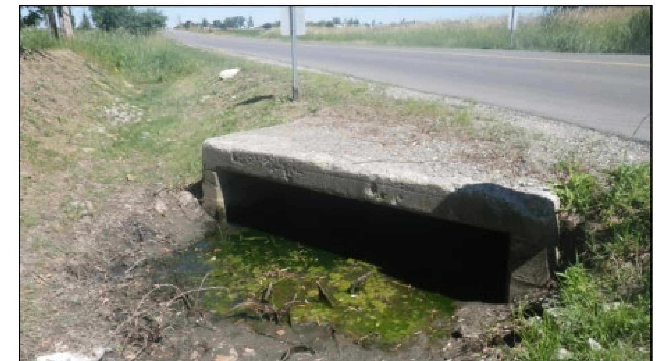
Reach R-6: Coleraine Drive culvert, extensive sedimentation impedes downstream flow along southside of Coleraine.
