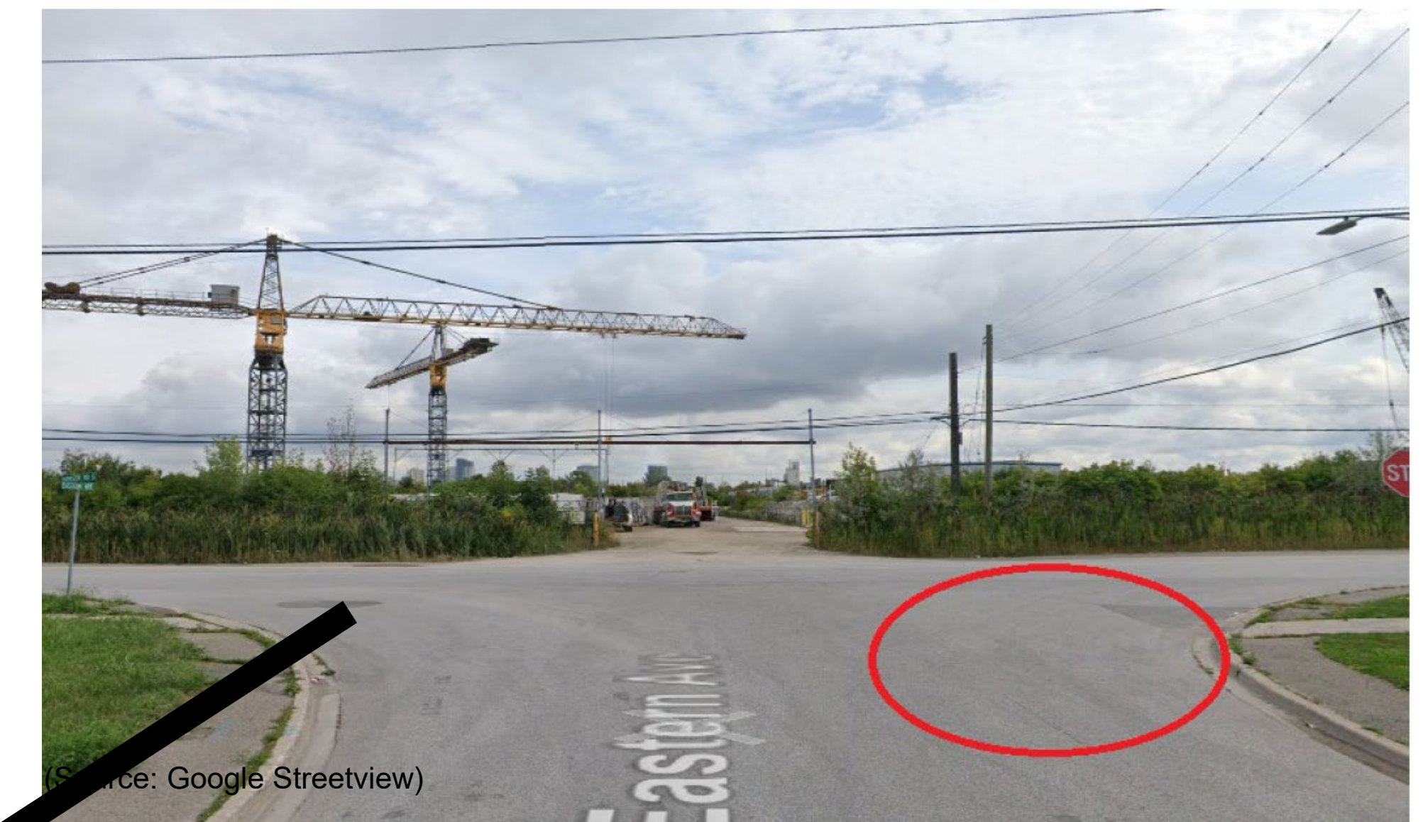
Missing pavement markings at the Eastern Ave / Hansen Rd intersection
