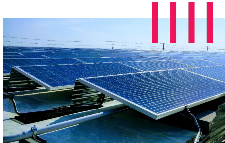
Roof-Mounted Solar Panels
