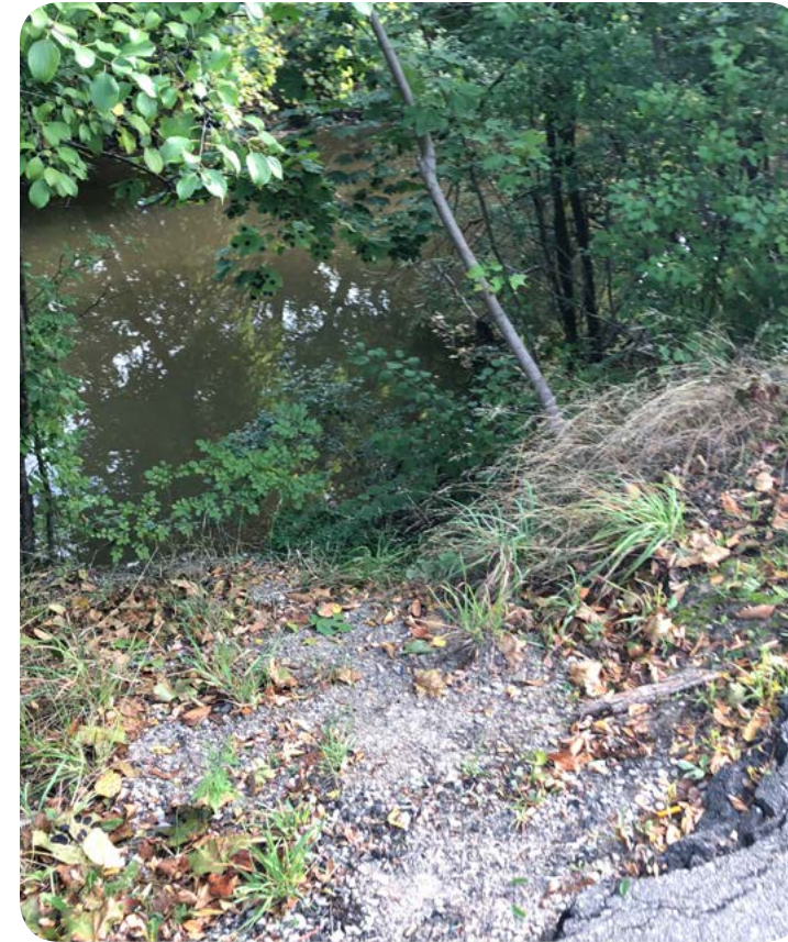
Creek Bank Erosion
