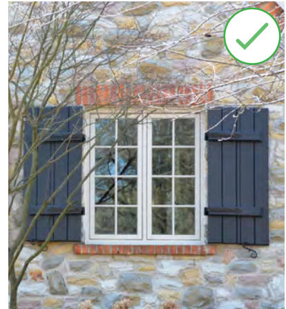
Figure 36. This photo shows operable storm shutters that are appropriately sized. (Source: City of Brampton)
