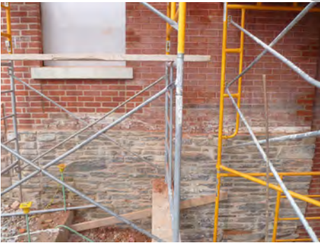
Figure 24. Ensure the historic finishes and textures of foundations are maintained. Repair or replacement should match the historic texture and finishes, as shown above. (Source: ERA)
