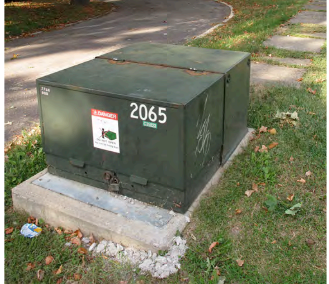
Figure 86. Installation of public utilities on Main Street South impact the heritage character of the streetscape. (Source: ERA)
