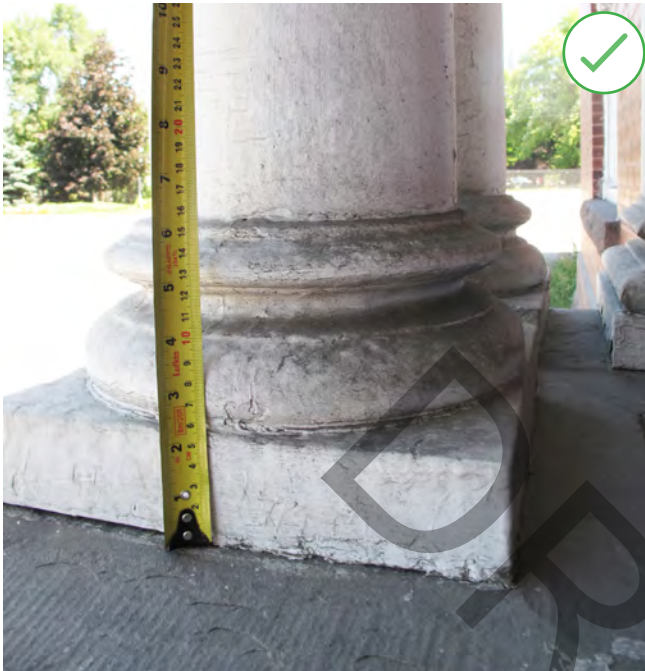
Figure 31. Completing detailed measurements of this column base was the first step in conserving this column. (Source: ERA)
