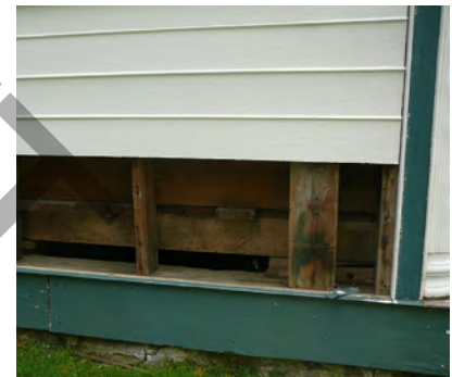
Figure 14. This project involved carefully removing part of the exterior wall in order to expose the interior structure and understand how to properly restore the exterior siding. (Source: ERA)
