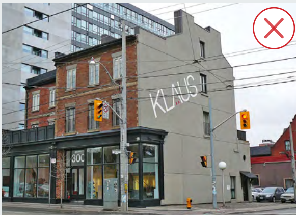
Figure 21. Detail and cut-away sample of the exterior wall showing the uniform texture of the synthetic stucco and the damaging to the masonry underneath. (Source: ERA)
