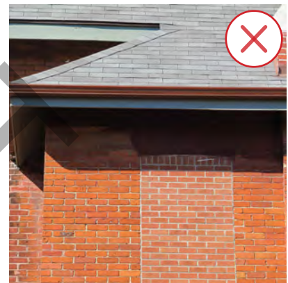
Figure 34. This photos shows a window opening bricked in. (Source: ERA)
