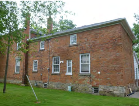
Figure 23. This photograph shows exposed foundation above grade being maintained as part of the building elevation. (Source: ERA)
