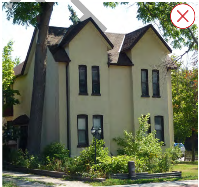
Figure 16. This house illustrates the application of new cladding material over historic brick, which detracts from the character of the building and conceals architectural details. (Source: ERA)
