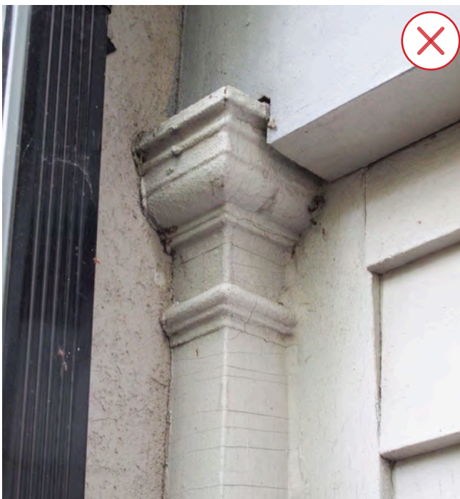
Figure 33. In this case, the decorative element was not considered when making changes to the building. As a result, it was partly obscured. This should be avoided. (Source: ERA)
