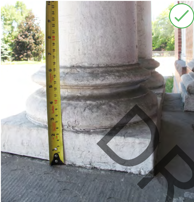
Figure 32. Completing detailed measurements of this column base was the first step in conserving this column. (Source: ERA)
