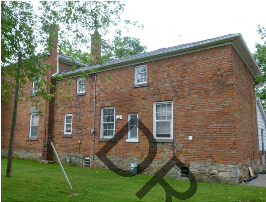
Figure 24. This photograph shows exposed foundation above grade being maintained as part of the building elevation. (Source: ERA)
