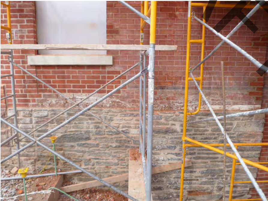
Figure 25. Ensure the historic finishes and textures of foundations is maintained. Repair or replacement should match the historic texture and finishes, as is shown above. (Source: ERA)
