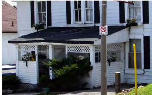
Unsympathetic porch addition.
