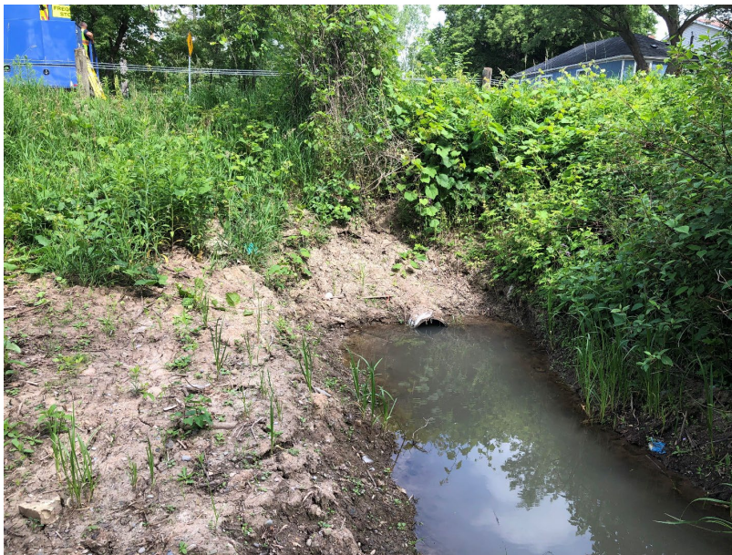
Photo 2-29: CSP culvert with inline check valve (OF_3980) at end of earth dyke section along Martins Blvd
