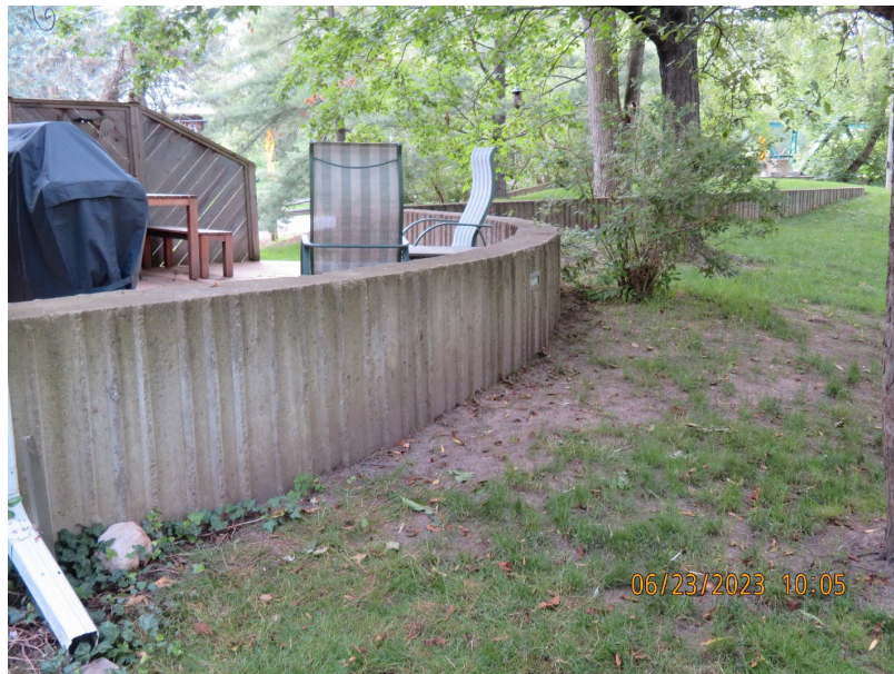
Photo 2-14: End of floodwall behind 7736 Churchville Road
