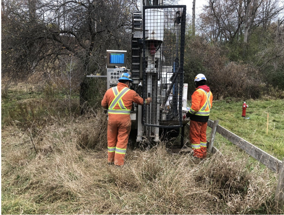
Photo 3-2: CPTu drill rig set-up at Churchville flood dyke (northern section on Churchville Road)
