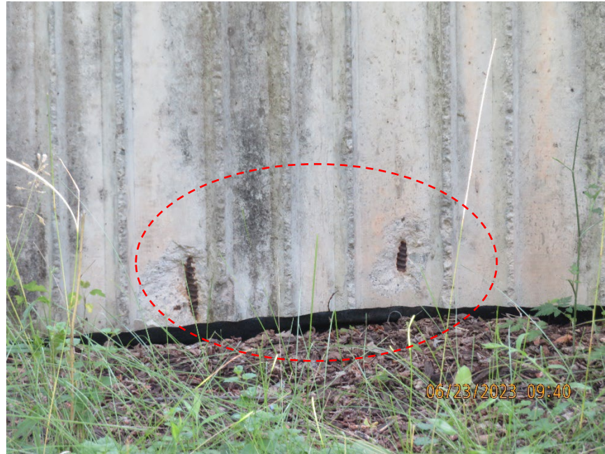
FIGURE 6-4: EXPOSED REBAR ON THE FLOODWALL
