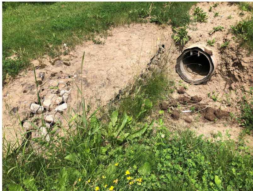
Photo 2-26: CSP culvert with inline check valve (OF_3979) near corner of Martins Blvd and Victoria Street
