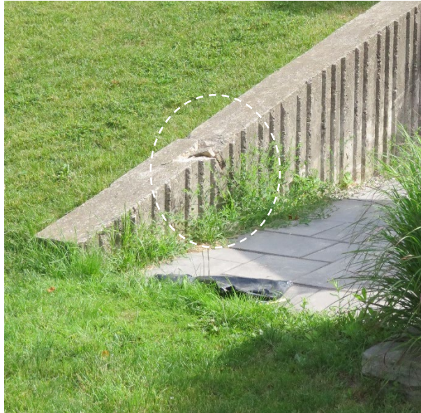
Photo 2-10: Crack in floodwall at wet-side toe
