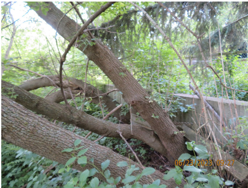
Photo 2-7: Larger/mature trees were observed growing near the concrete floodwall
