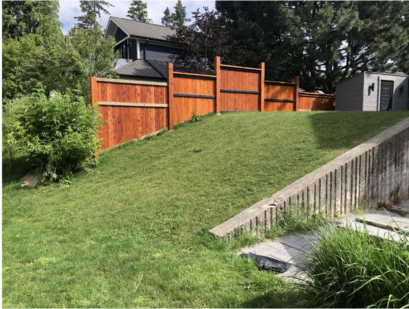
Photo 2-18: Wet side slope of dyke flanking north side of 7764 Churchville Road (looking north)
