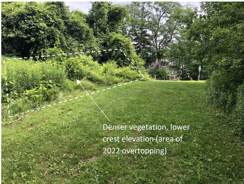
Photo 2-24: Wet side slope of dyke at Segment 4, near box culvert (area of 2022 overtopping)
