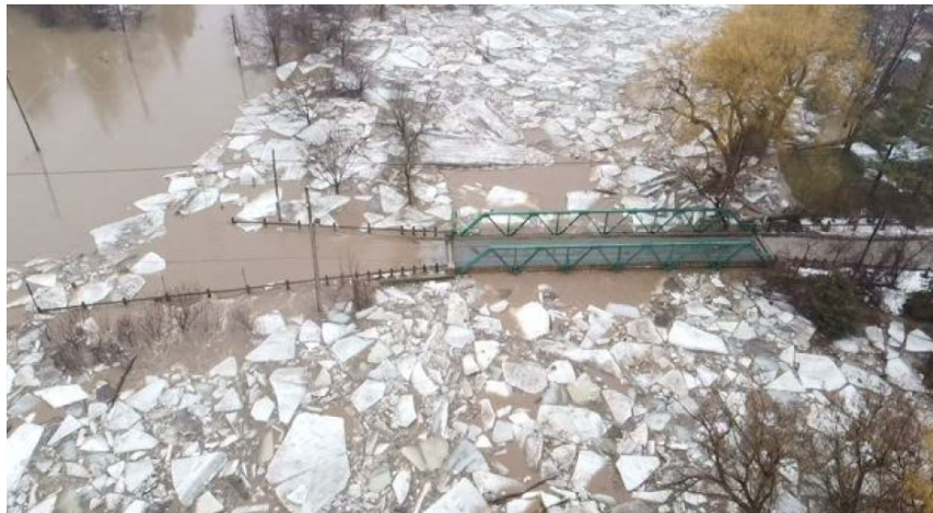
Photo 1-1: Churchville Road Bridge following February 2022 Flood Event
