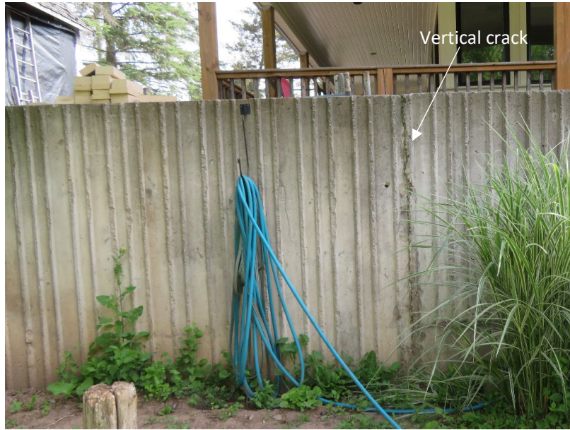
Photo 2-4: Vertical crack in concrete wall
