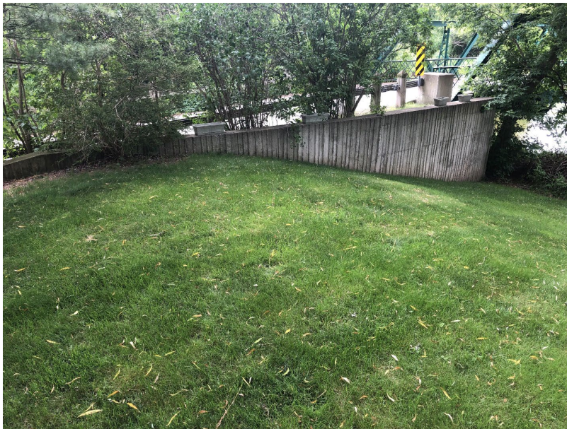
Photo 2-20: Crest and wet side slope of berm west of bridge, looking south
