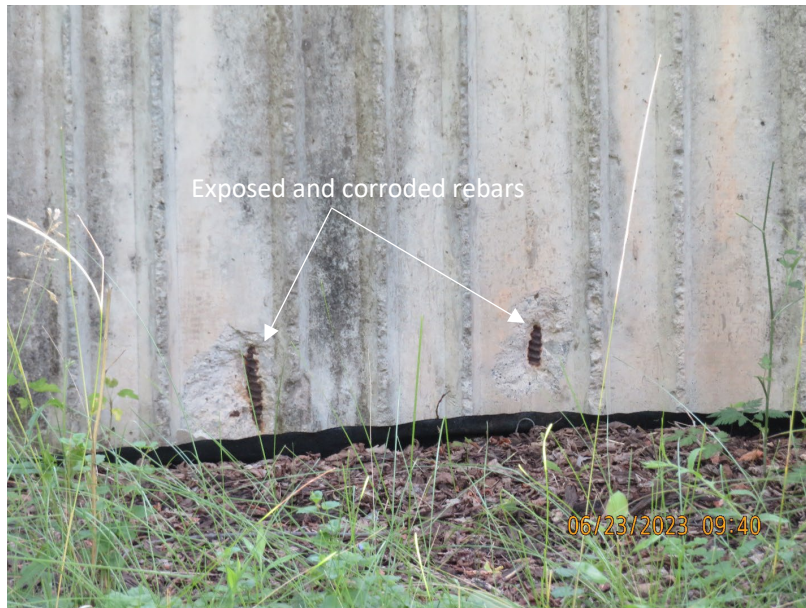
Photo 2-5: Exposed and corroded rebar
