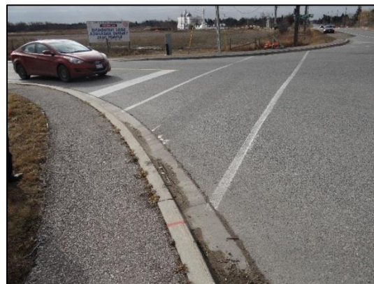
Figure 19: Lack of Pedestrian Infrastructure (Clarkway Drive and Mayfield Road)
