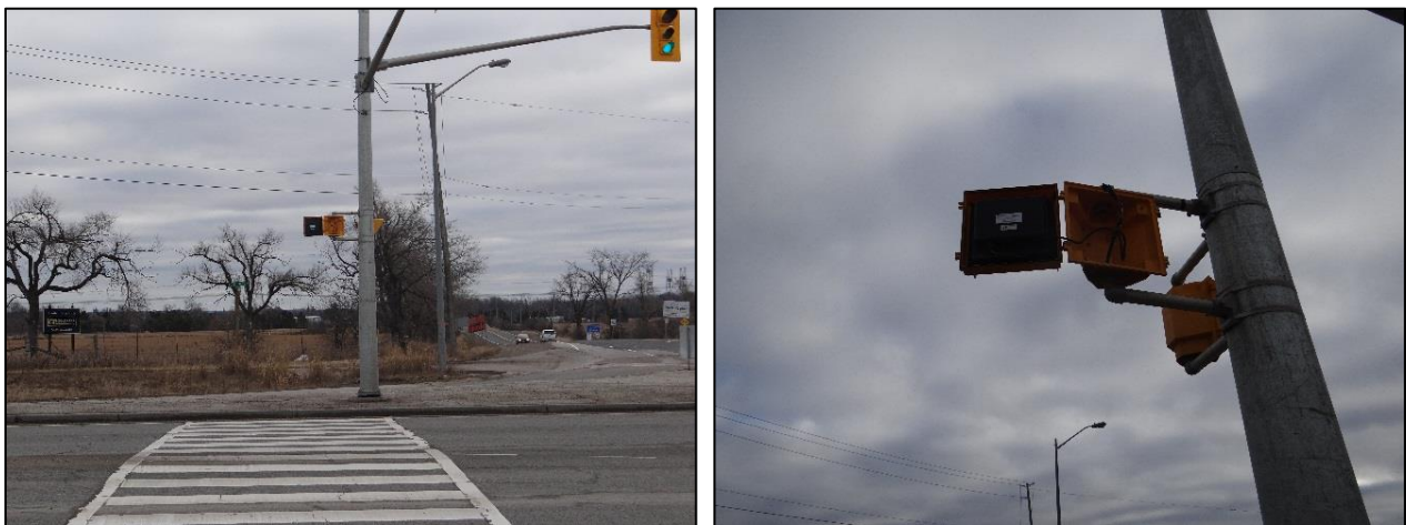
Figure 29: Broken Pedestrian Signal Head (Countryside Drive and Regional Road 50)
