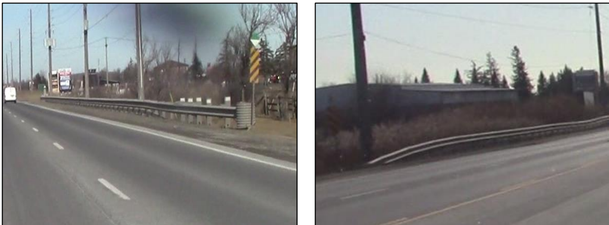
Figure 35: Missing Crash Cushion along Regional Road 50
