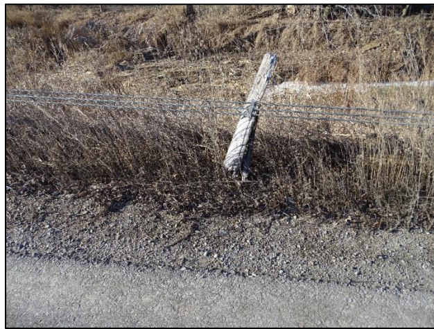
Figure 20: Damaged Cable Guide Rail along the Clarkway Drive
