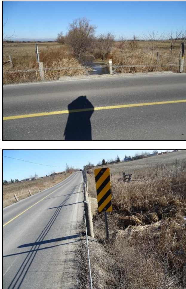
Figure 33: 3-Cable Guide Rail along Countryside Drive
