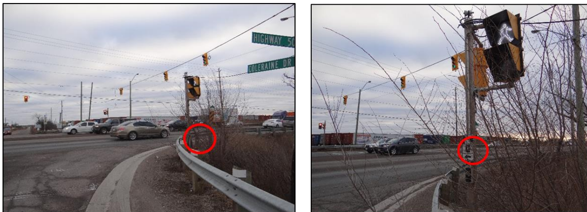
Figure 10: Obstructed Pedestrian Push Button (Coleraine Drive and Regional Road 50)
