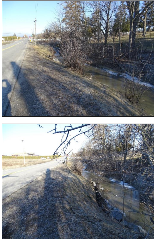
Figure 22: Inadequate Steel Beam Length along the Clarkway Drive
