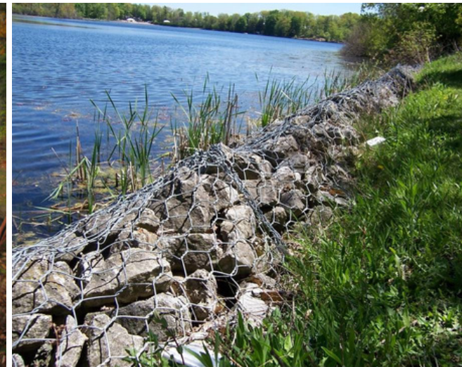
Failing Gabion Baskets
