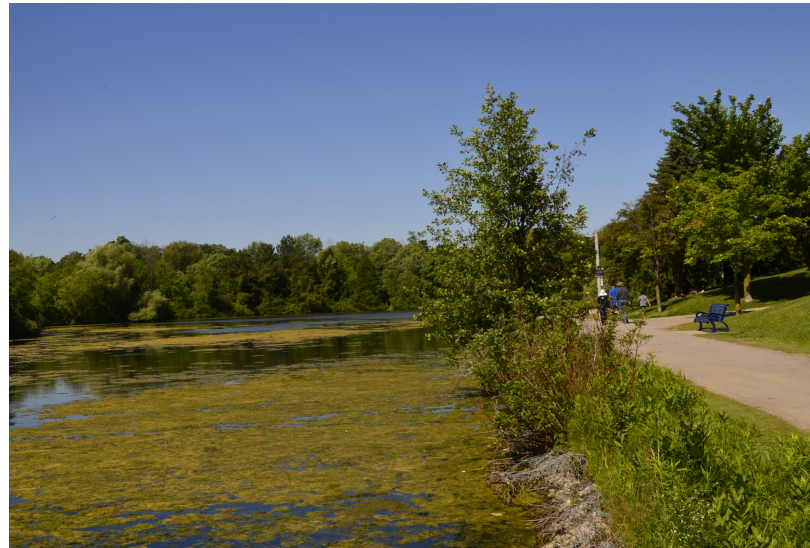
Eroded Shoreline and Failing Gabion Baskets
