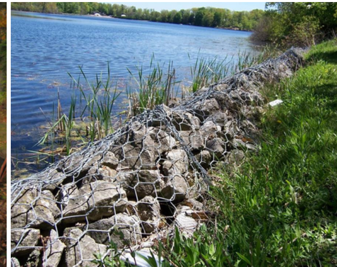
Failing Gabion Baskets
