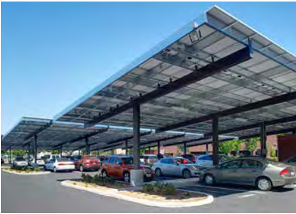
Solar parking lot canopies.
