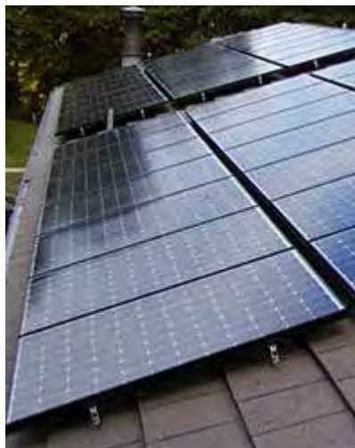
Roof mounted photovoltaic system
